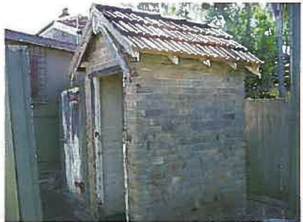
Figure 4.21 On-site redundant W.C.
